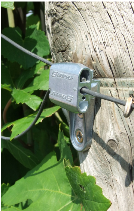
VIT-S Kit - Installed on wooden post
